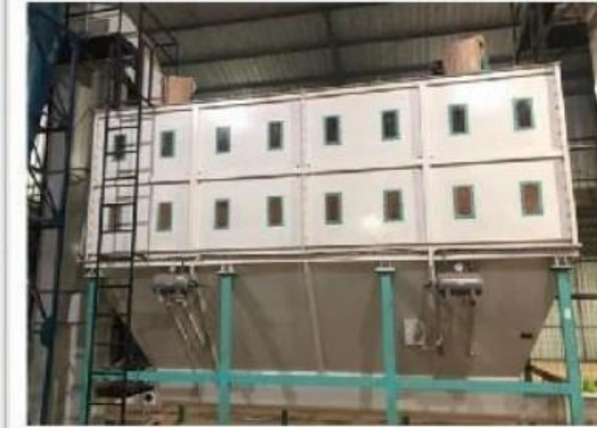
BUFFER STORAGE / SILO
